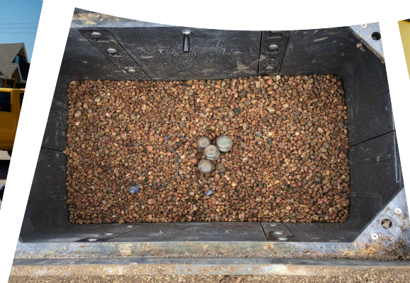
Capped Microduct in Vault
